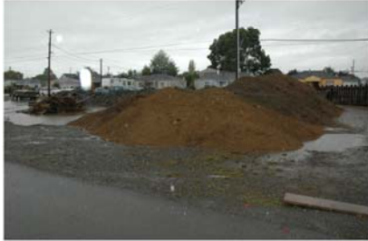
Picture 4. Un-protected stockpile.
