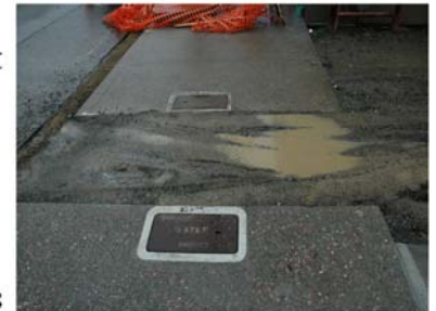
Picture 2. Sediment near failed wattles.
