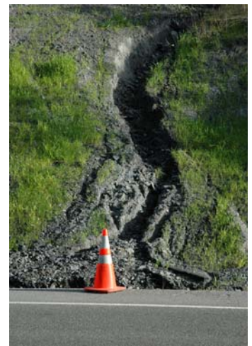
Figure 7b. Hwy. 299 erosion.
